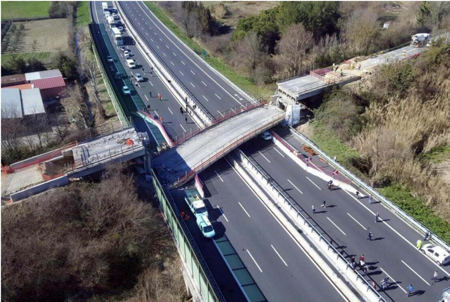
A bridge that collapsed onto the A14 motorway near the central Italian city of Ancona EPA
